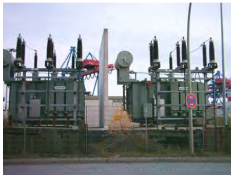
Figure 20.19 Power is distributed over large distances at high voltage to reduce power loss in the transmission lines. The voltages generated at the power plant are stepped up by passive devices called transformers (see Transformers ) to 330,000 volts (or more in some places worldwide). At the point of use, the transformers reduce the voltage transmitted for safe residential and commercial use. (Credit: GeorgHH, Wikimedia Commons)
